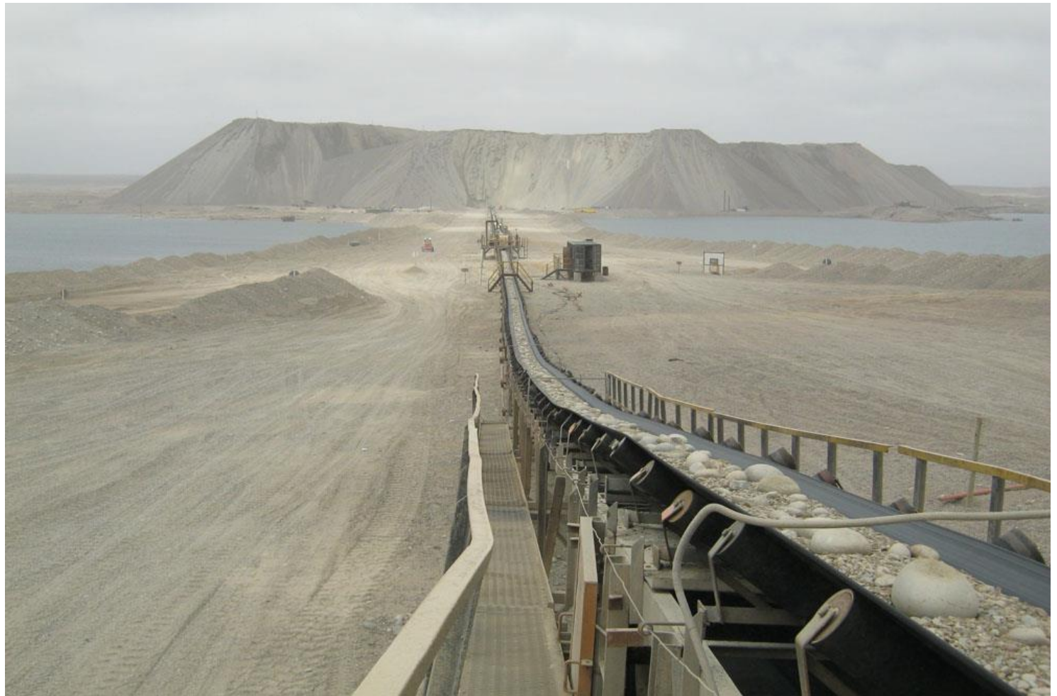
NAMDEB: MA1 material handling
